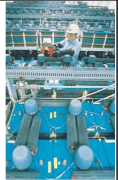
The world's largest battery energy storage plant (dismantled in 1996) connected over 3000 large lead-acid batteries in 8 strings at 1000 V each with a capability of 10 MW of power for 4 hours. Charged up at night, the batteries were then put to use during peak power demands on the electrical system. (Courtesy Southern California Edison Company)
